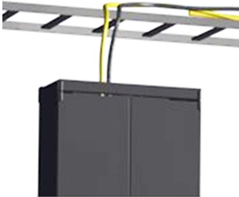
Figure 32. Ladder Racking Above OMX Splice Cabinet
